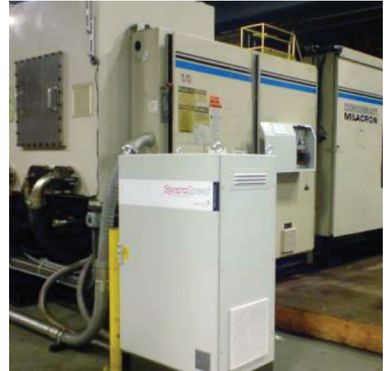
SyncroSpeed 135 HP 2-motor system installed on a Cincinnati 723t.
