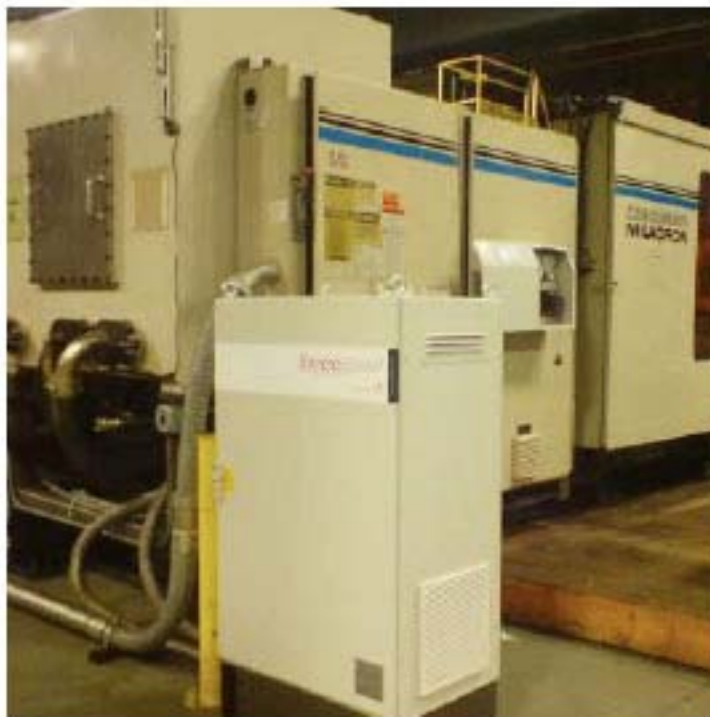
SyncroSpeed 135 HP 2-motor system installed on a Cincinnati 725t
